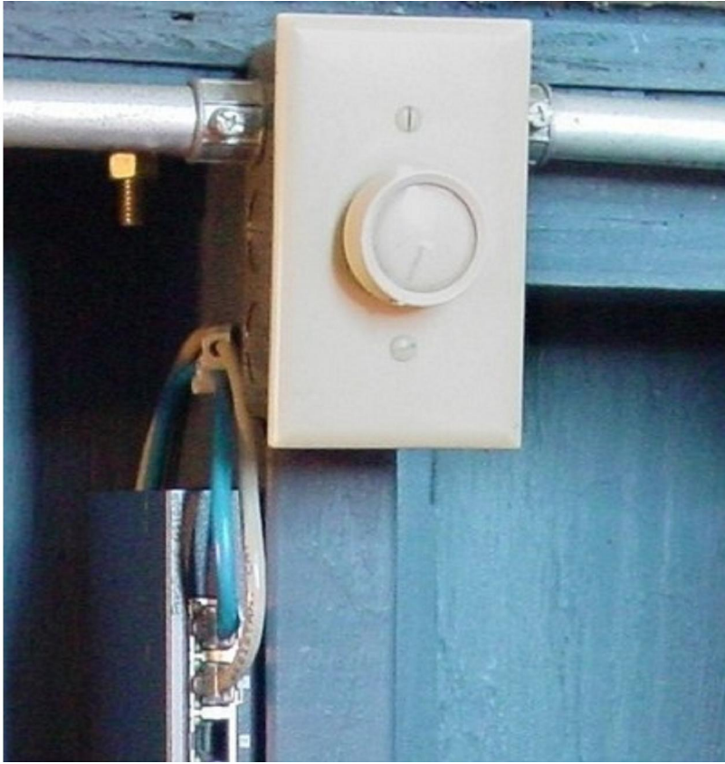
This is also a dimmer for the white lights.
