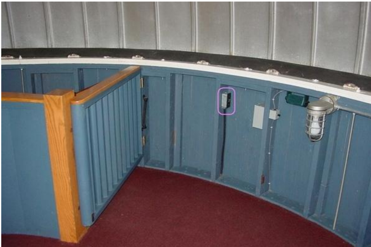
Top of stairs light switch by gate.
