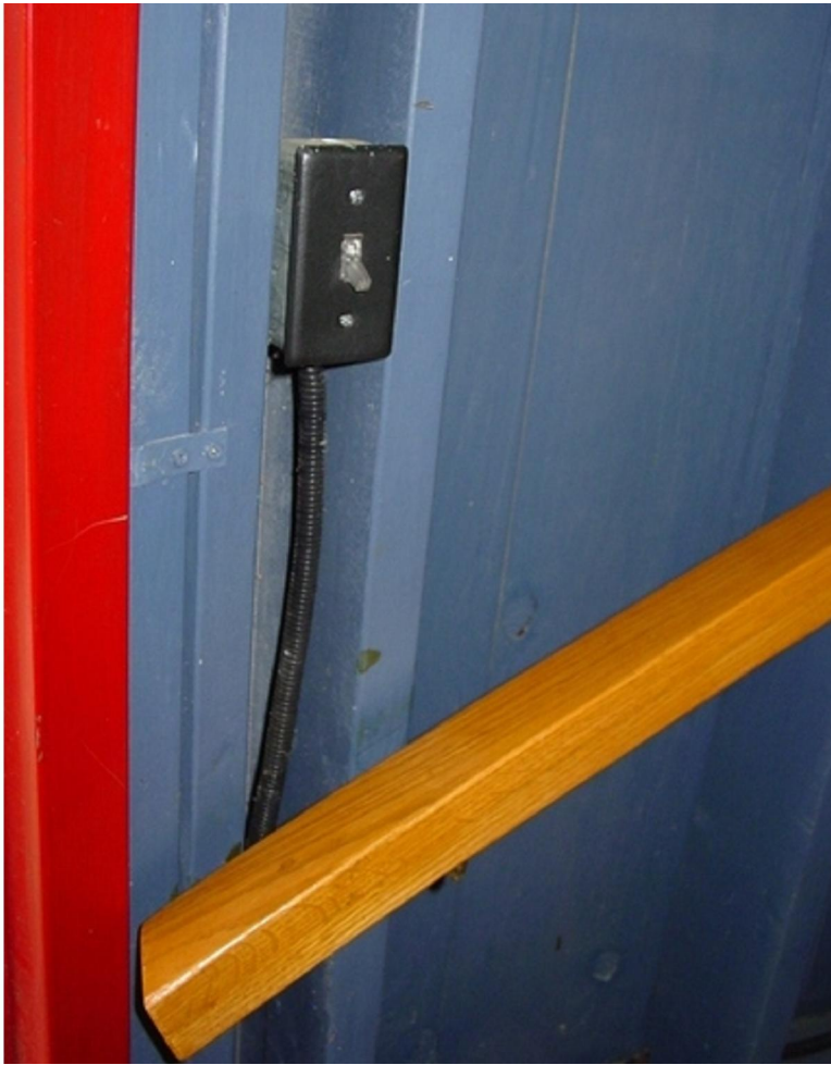
Bottom of stairs light switch, left side of door.
